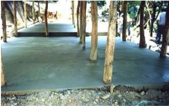
The first of 15 concrete floors that are being poured in Guatemala. People should not have to live on dirt where disease spreads.
