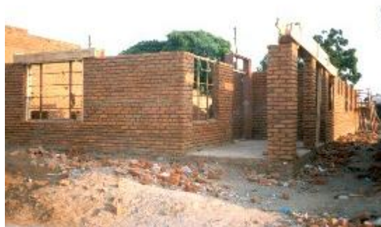
The Malakia Clinic and Birthing Center under construction. This facility being built with the support of hundreds of volunteers. Photo taken October 12, 2000.
